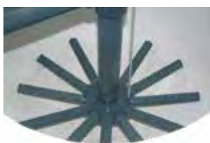
Collector arms detail
