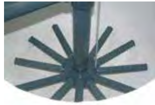
Collector arms detail
